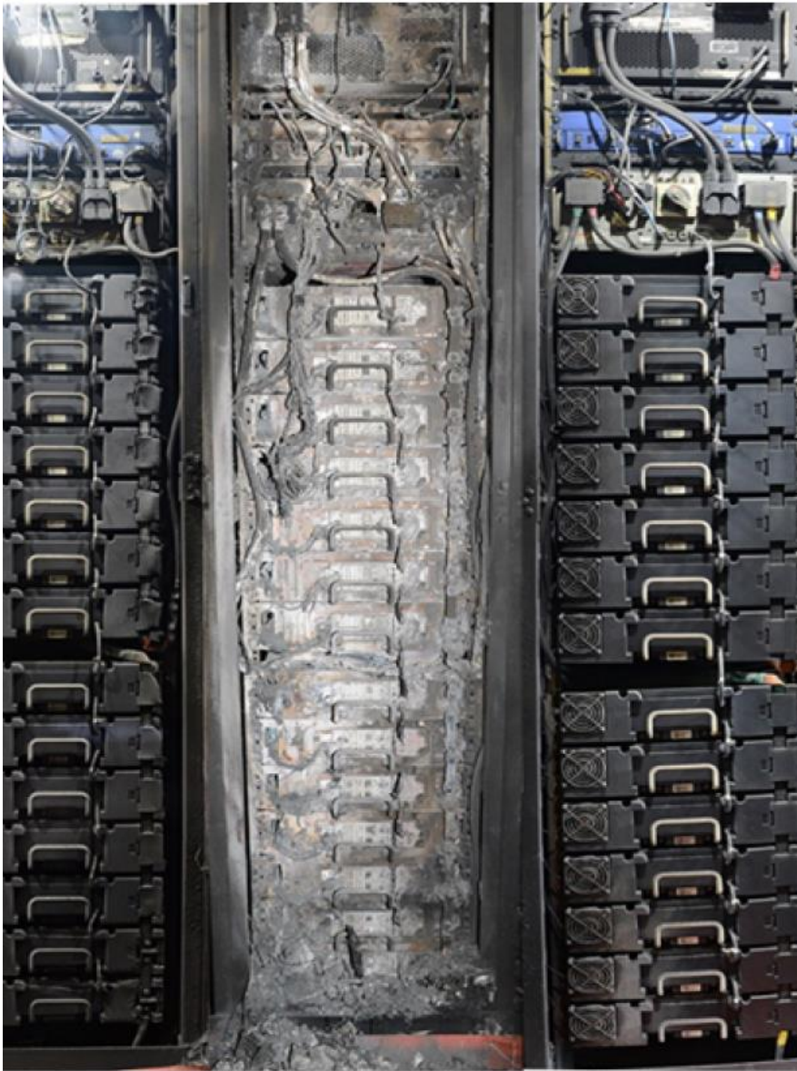
Rack 17 Rack 15 Rack 13
